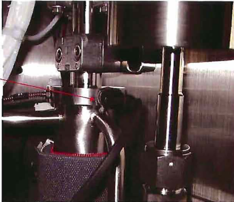
Figure 34. Thermostat on Expansion Chamber 2.
