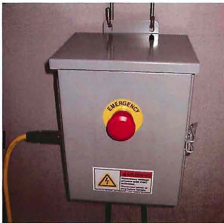
Figure 9. Pump controller box.
